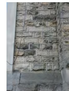
105 Union Street, insensitive repointing
