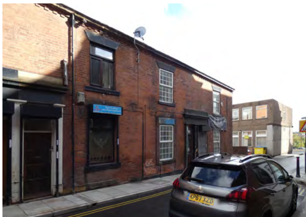
Plate 9.25 Poor quality alterations including modern windows, roller shutters and signage to southern end of terrace group
