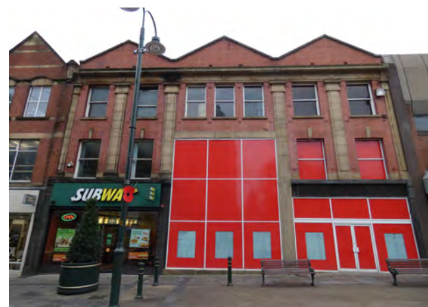
Plate 9.16 Poor signage and shopfronts within proposed extension causing harm to overall appearance of building which makes a positive contribution to the conservation area
