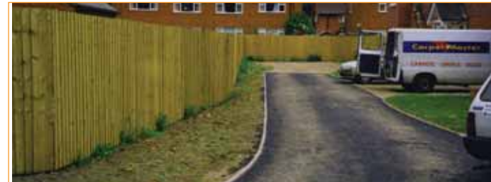
This poor quality close-boarded fence will require a high level of maintenance to ensure it provides a secure boundary
