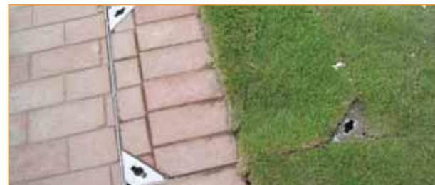
Coordinating services and landscape can help to avoid problems like this
